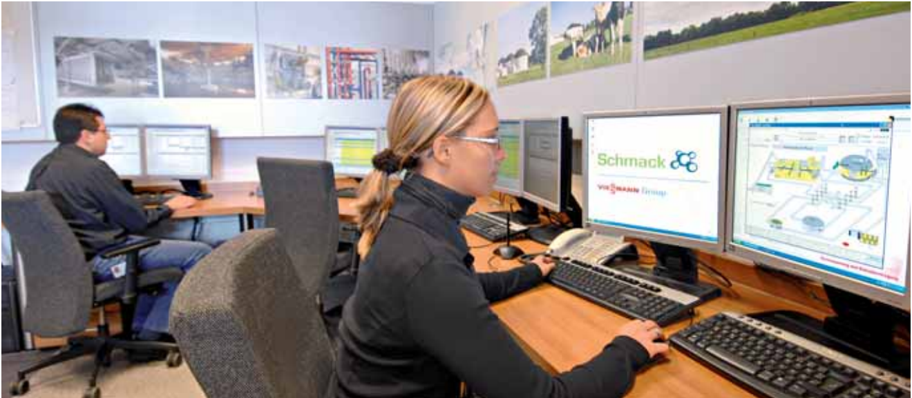
EUVIS control centre
